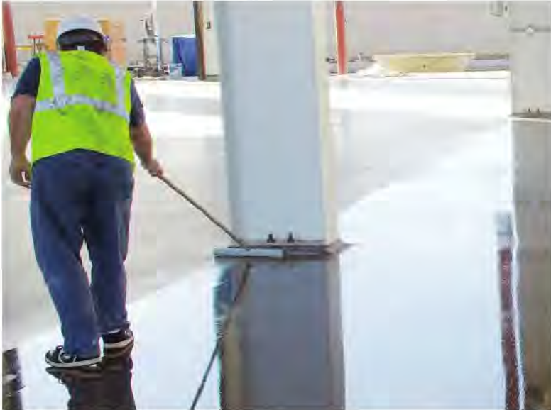
Use of chemistry that is pH-neutral and does not require rinsing, coupled with equipment that is environmentally responsible, yields a polished concrete floor created with lower downtime.
