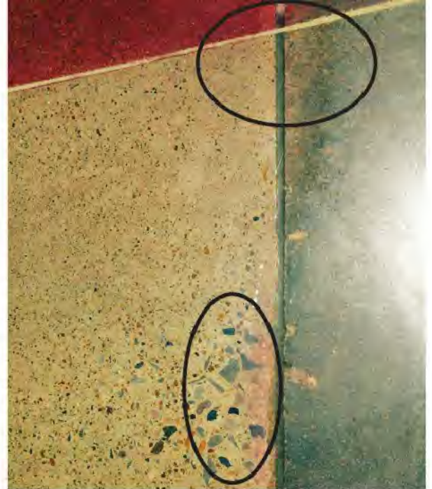
This photo shows two common pitfalls: color misapplication and slab curl with the resulting uneven joints, elevated by Type G concrete.
