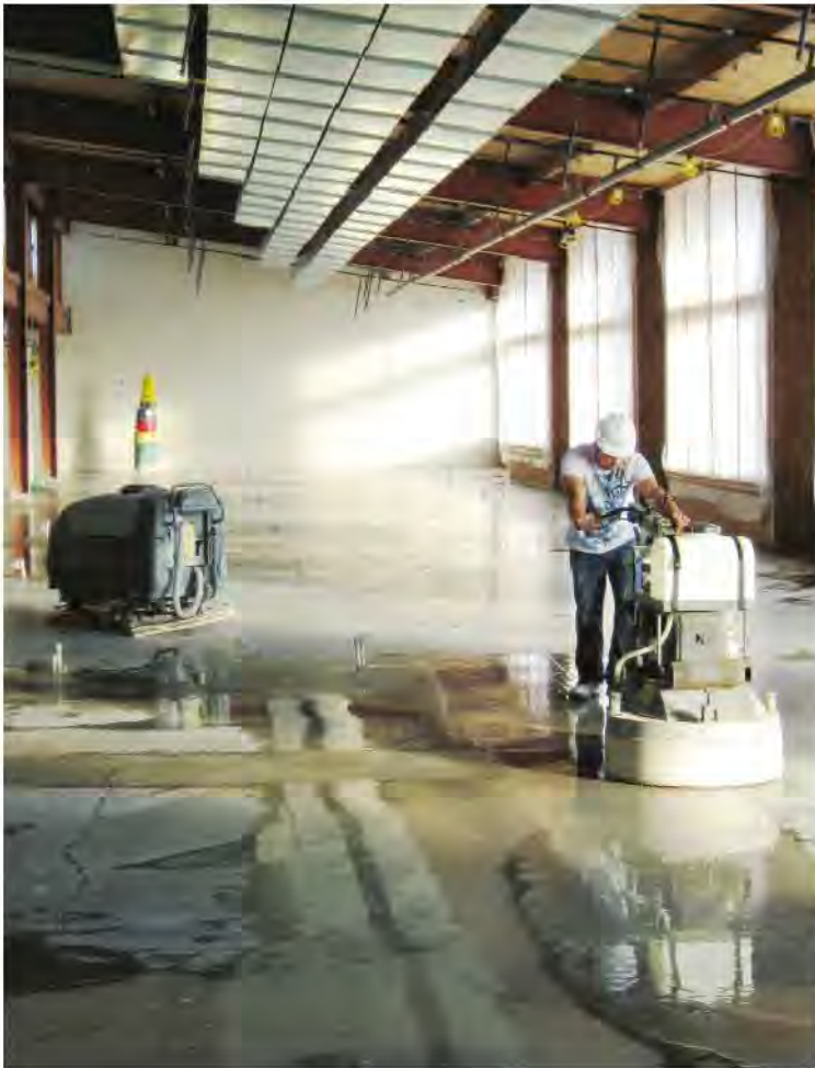
Processing a floor 'wet' can improve ambient air quality; using heavy-duty grinding equipment allows for the floor to be processed throughout—from grind and hone to final polish.
