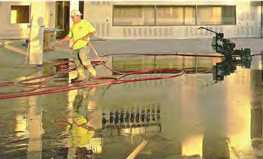
The grinding and honing process should be done wet using reactive, non-water-soluble, pH-neutral chemistry to minimize silica dust contamination.
